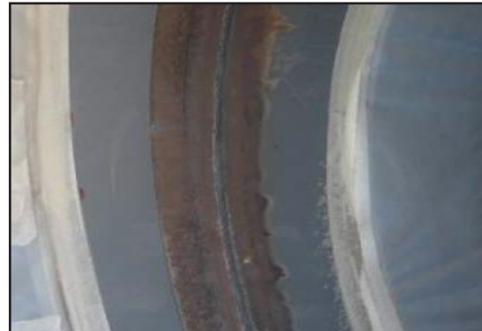
Internal uncoated girth weld
